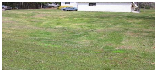
Patches of lush green grass over a drain field or septic tank could be a sign of a failing system.
