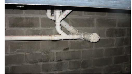
A certified evaluator will check the interior plumbing to make sure it is properly connected to the septic system and is without leaks.
